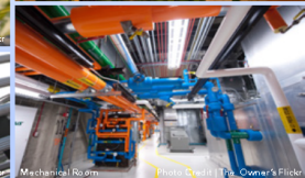
Mechanical Room Photo Credit | The Owner's Flickr
